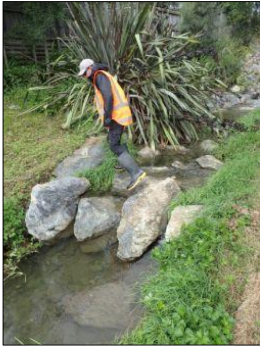
Figure 10. Large rocks downstream Hill street culvert
