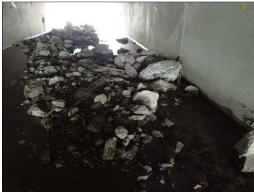
Figure 15. Rocks and gravel build up in Concordia Lane culvert
