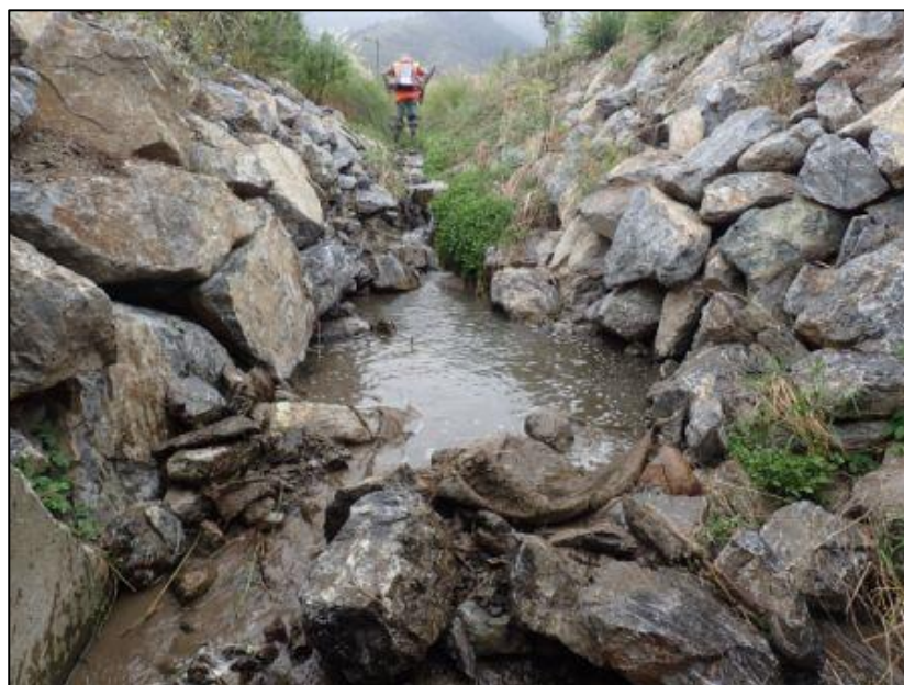
Figure 13. Uplifted filter cloth partially cleared
